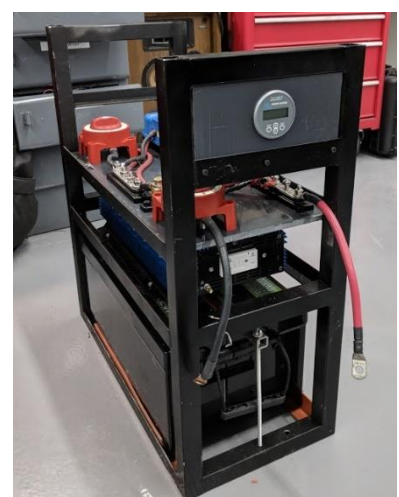
Figure 38) Fabricated and populated electrical containment box
